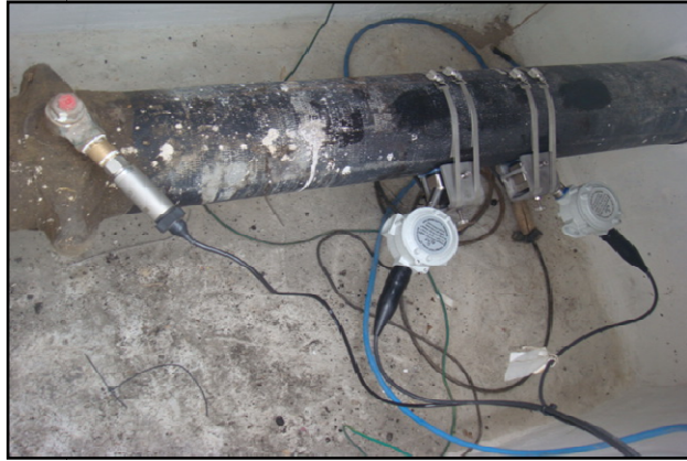
Fig. 2-6: Water flow and pressure sensor fitted on a water pipe (Hussain, Zainal, Elmedany, & Fakhr, November 2012)
