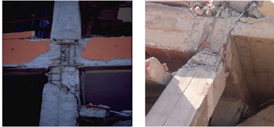
Figure 1.2 Typical BCJs during earthquake in Turkey (1999) and Algeria (2003) (Ajmal, 2016)
